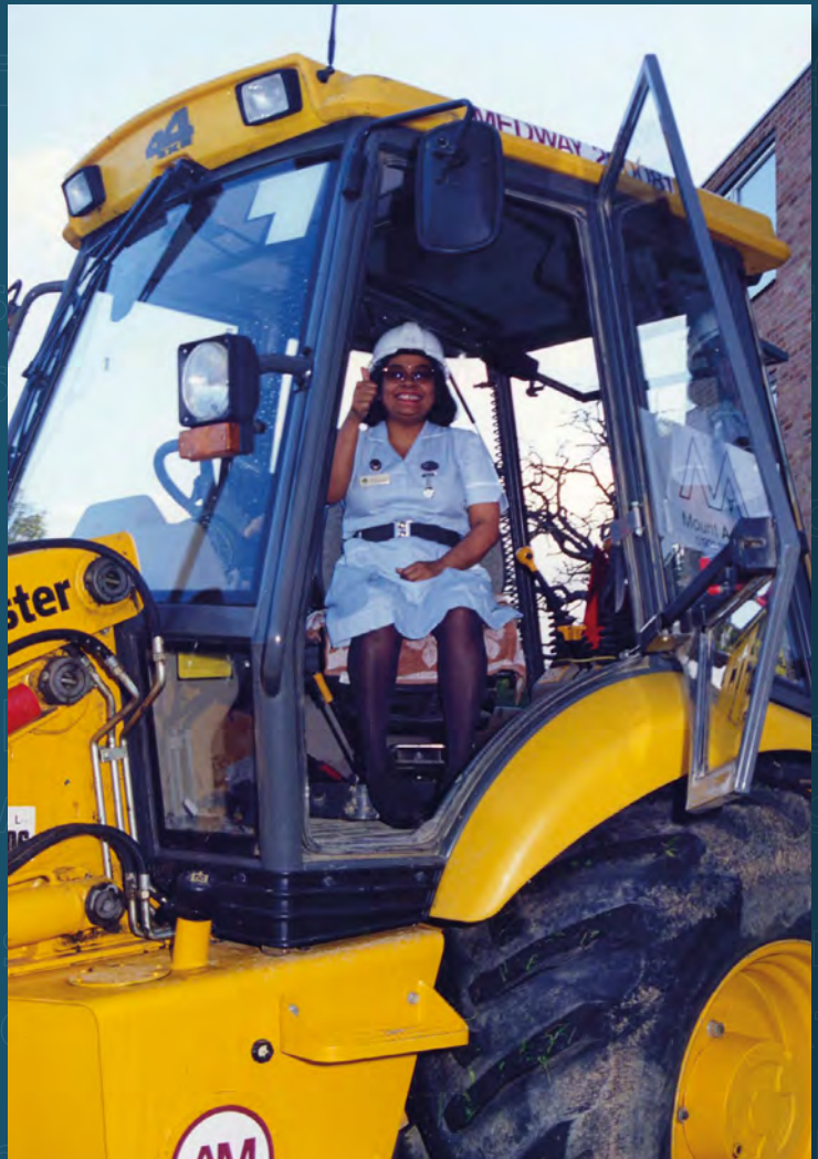
Senior Nurse Shirley Patel appears eager to start the demolition of old residential accommodation at Queen Mary's Hospital Sidcup in 2000.
